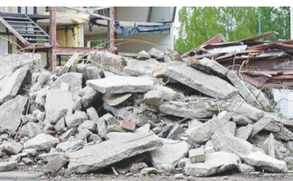
ETAWAH, Oct 28 (Agencies): A 22-year-old labourer was killed when a portion of a dilapidated building was pulling down fell on him in Uttar Pradesh's Etawah, police said on Saturday.
